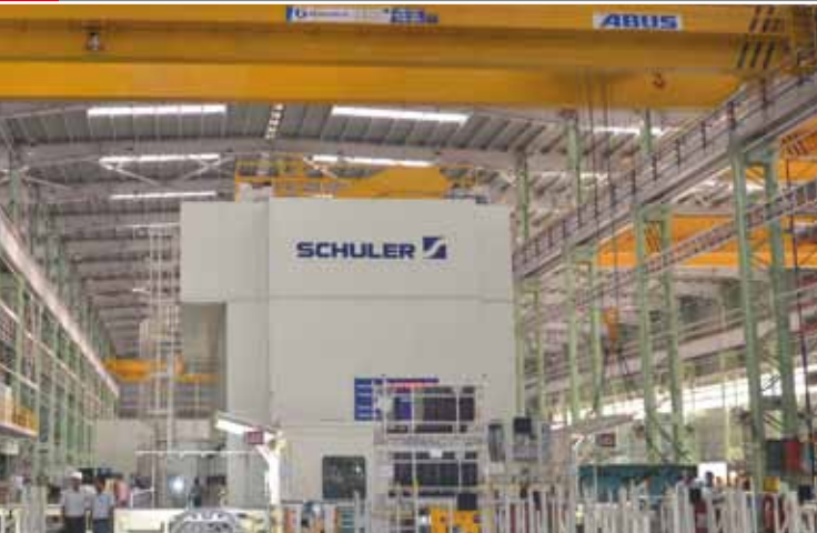
CHAKAN PLANT: The completely modular and flexible Schuler press line, one of three such machines in the world.
